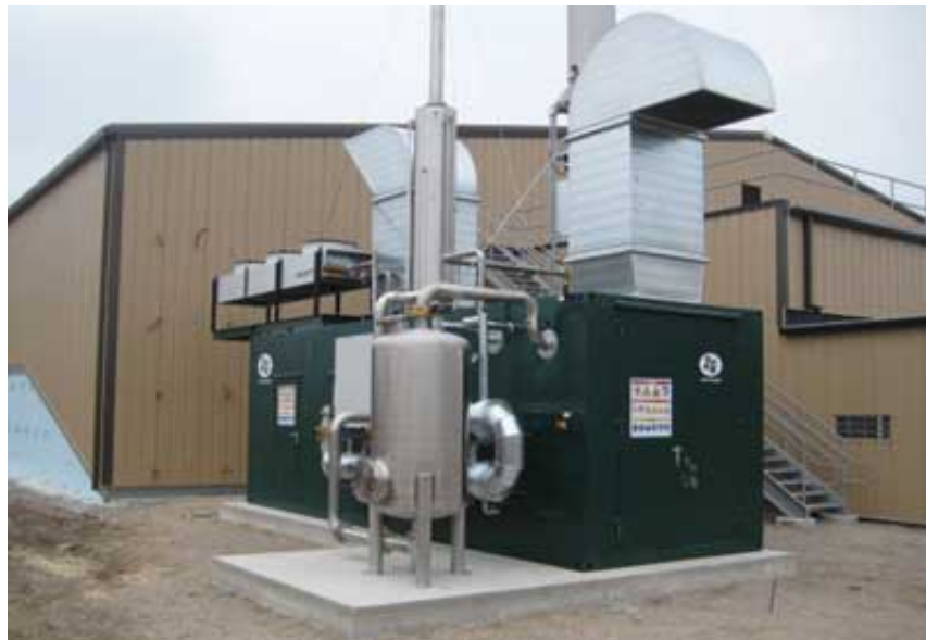
2G-Cenergy CHP unit outside BioFERM digester building Source: 2G-Cenergy
